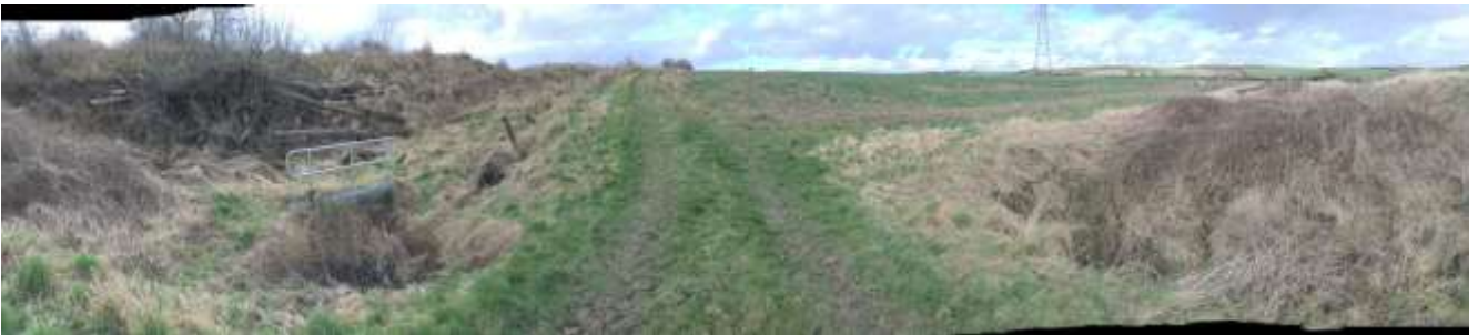
Figure 3.5 : Existing Watercourse 2 flowing right to left, piped under the existing farm access prior to been conveyed under the railway in a culvert (culvert headwall with metal barrier on top to left of photo)
