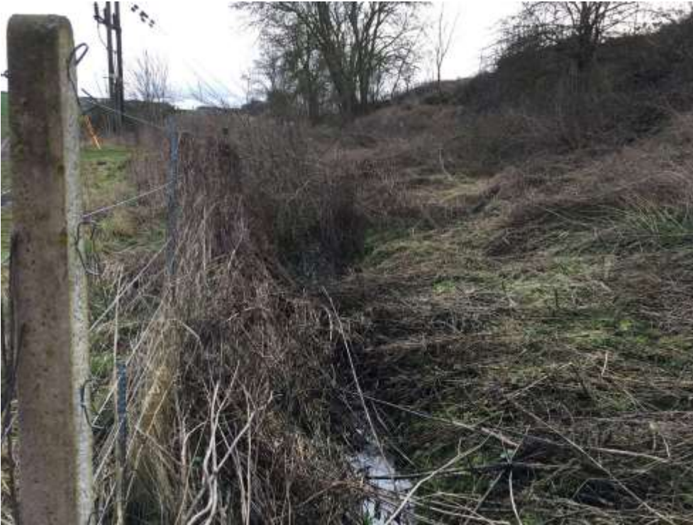
Figure 3.4 : Existing watercourse running parallel to railway, connects with existing watercourse 1 at the railway culvert
